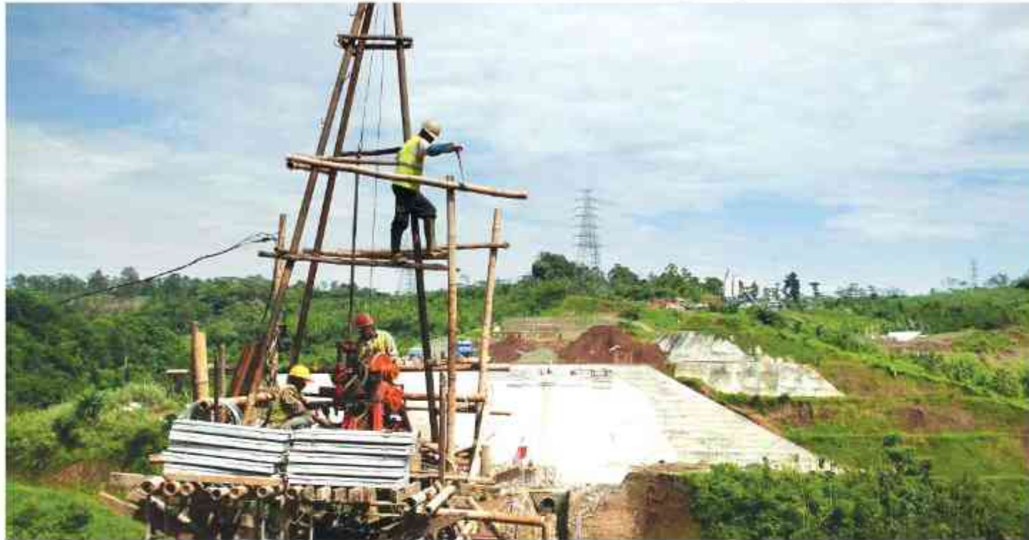
Seepage Measurement Jatiluhur Dam Project, Purwakarta-West Java
