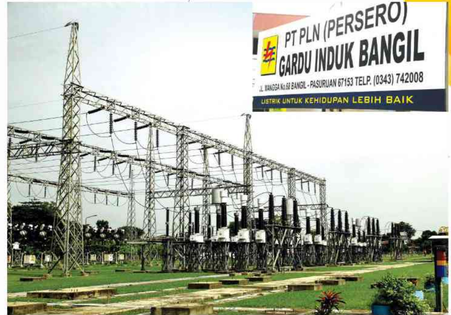
Bangil 150 KV Gis Sub Station, Bangil-East Java
