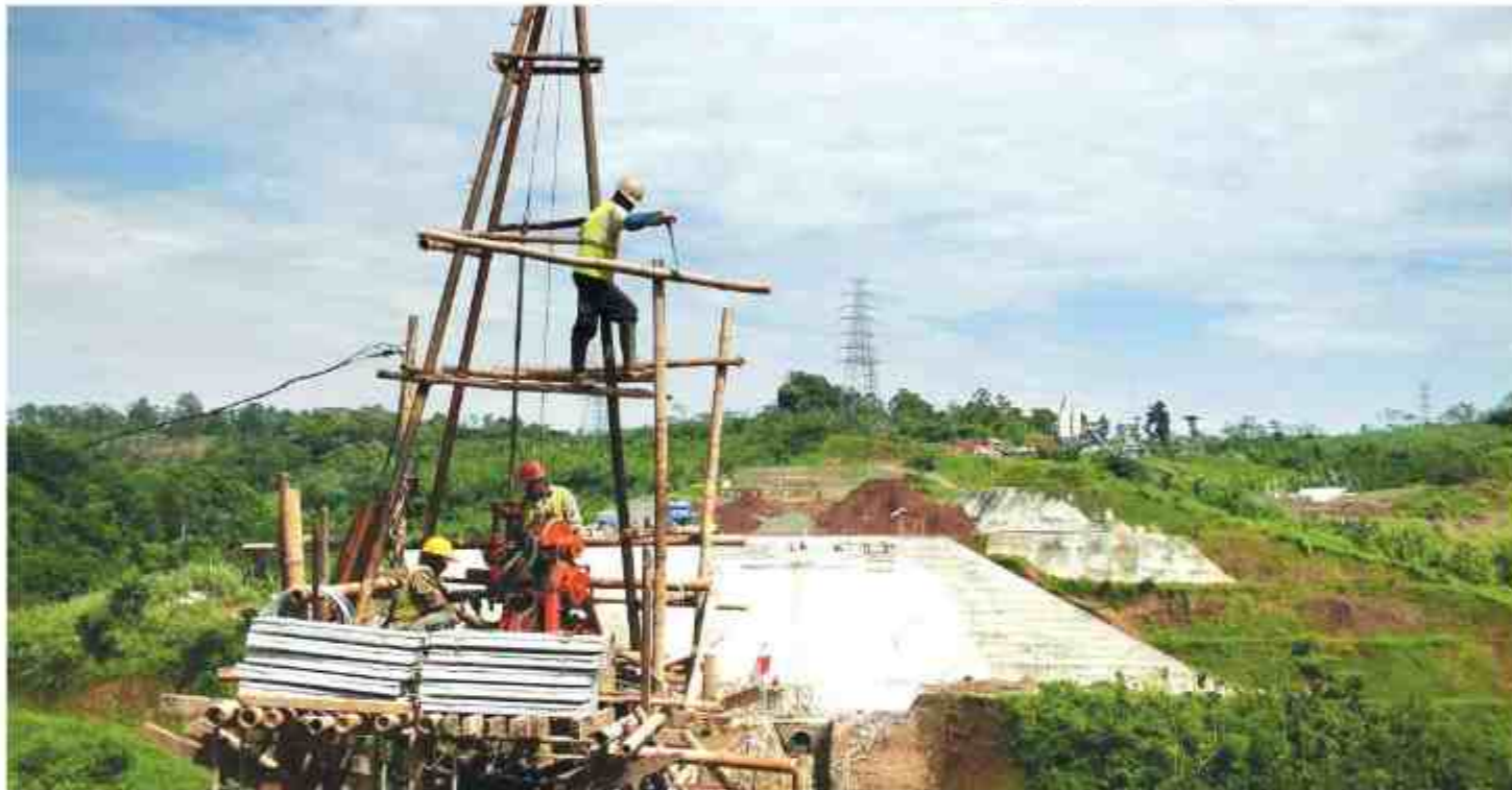
Seepage Measurement Jatiluhur Dam Project, Purwakarta-West Java
