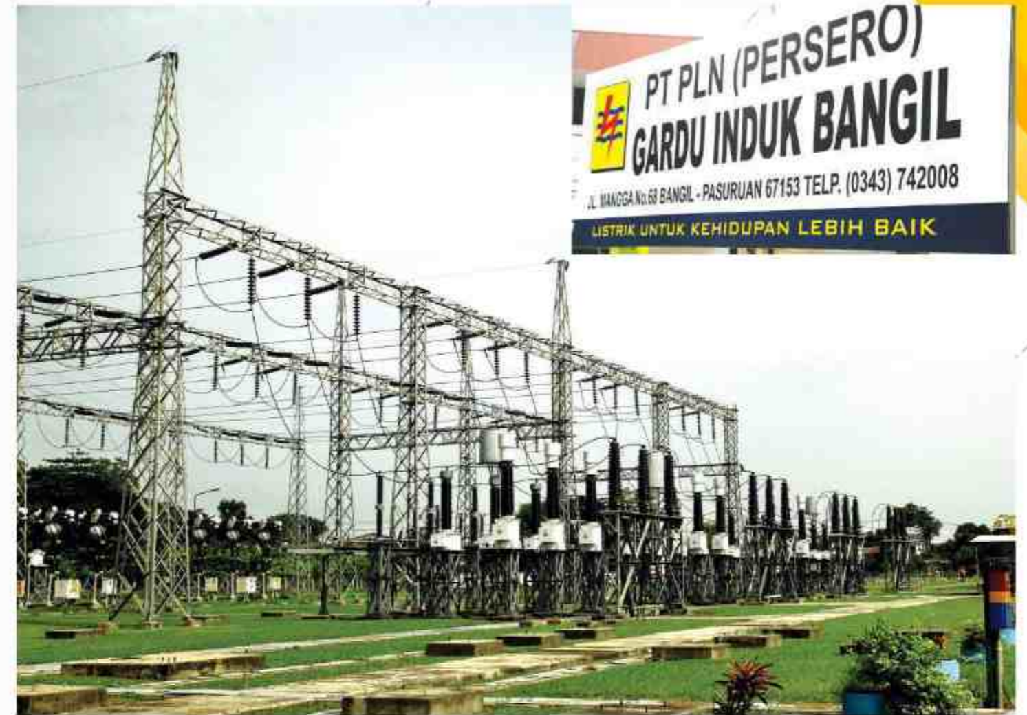
Bangil 150 KV Gis Sub Station, Bangil-East Java
