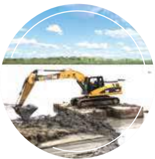
HOT MUD DISASTER MITIGATION
