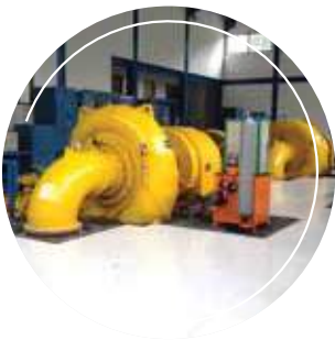
NDUNGA MICRO HYDRO POWER PLANT
