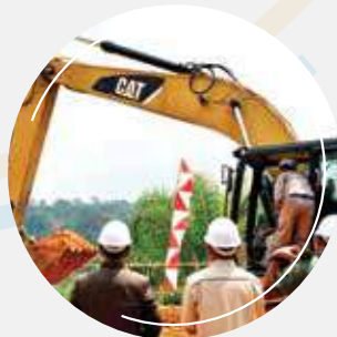
5 September | September 5 Ground Breaking PLTM Padang Guci, Bengkulu Ground Breaking hydropower Jar Padang, Bengkulu
